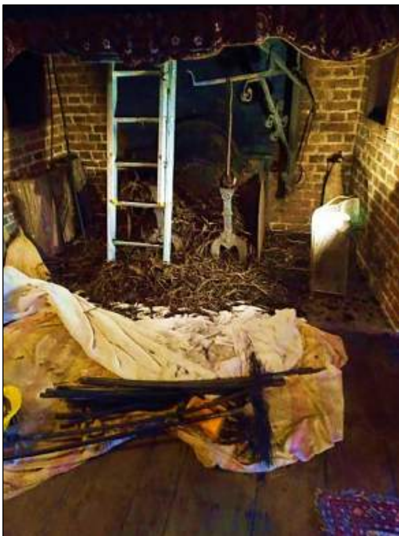
24 Nesting material for removal from the parlour Chimney
